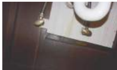
Water for hall bathroom sink was turned off at valves in cabinet. No immediate evidence of leakage when faucet was tested. Inspector turned water back off at cut-off valves. Recommend review with owner.
