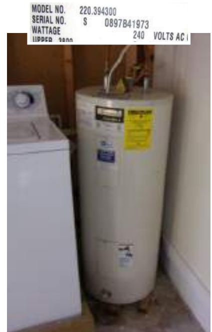
Electric water heater was in garage. Unit was 22 years old. Typical useful life is 14-18 years. Unit functioned when tested.
