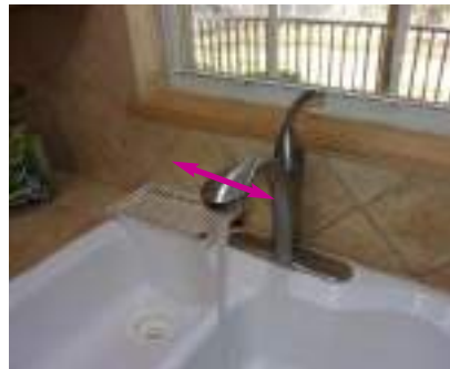
Kitchen faucet was difficult to move from side to side.
