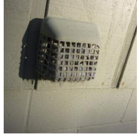
Recommend cleaning dryer duct.
