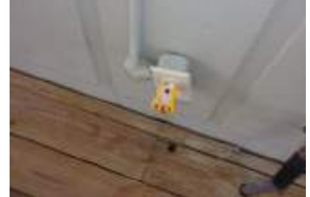
No power at one of the outlets on back porch.
