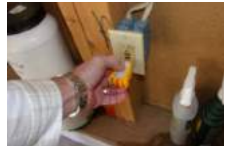
GFCI outlet in garage did not trip when tested.
