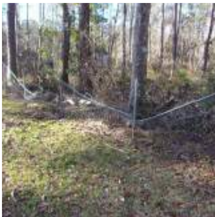
Significant damage at chain link fence.
