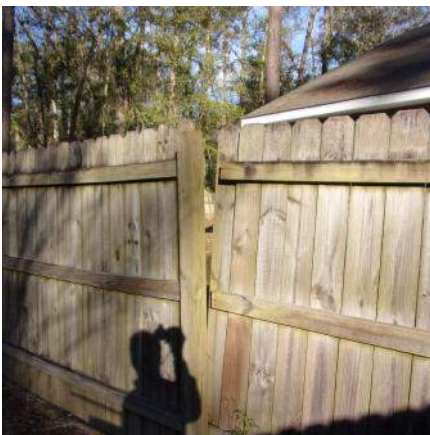
Loose wood fence panel at right side.
