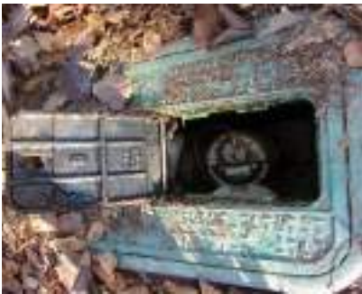
Main water shut-off at meter box in front.
